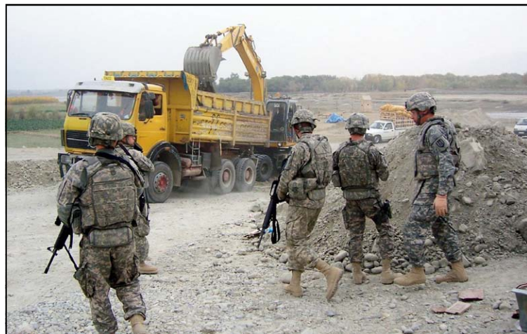
SOLDIERS from the 372nd Engineer Brigade survey and design team wait to perform a reconnaissance of a construction site.
