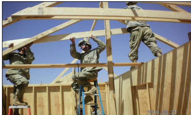
SOLDIERS from the 92nd Engineer Battalion (construction) Fort Stewart, GA, construct SEA-huts at Forward Operating Base Sharana Paktika province, Afghanistan.
